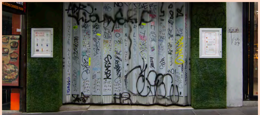
Figure 71 Solid metal shutters present poorly to the public realm when closed and are prone to graffiti and damage.
