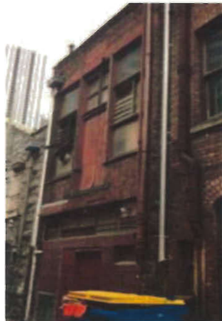
Photo 2: Altered rear wall
