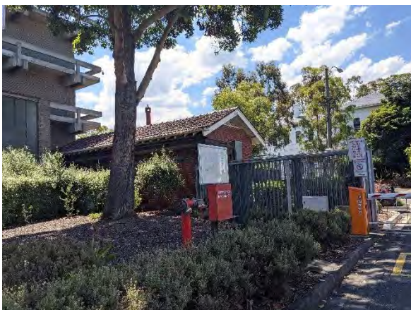
Figure 164. Northern substation. (Source: GML, 2023)
