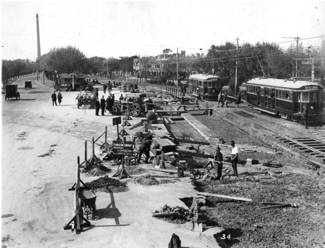
Figure 3.66 Electric tramlines being installed on St Kilda Road, looking towards the city, c.1925. (Source: State Library Victoria, Accession No. H40275/22)
