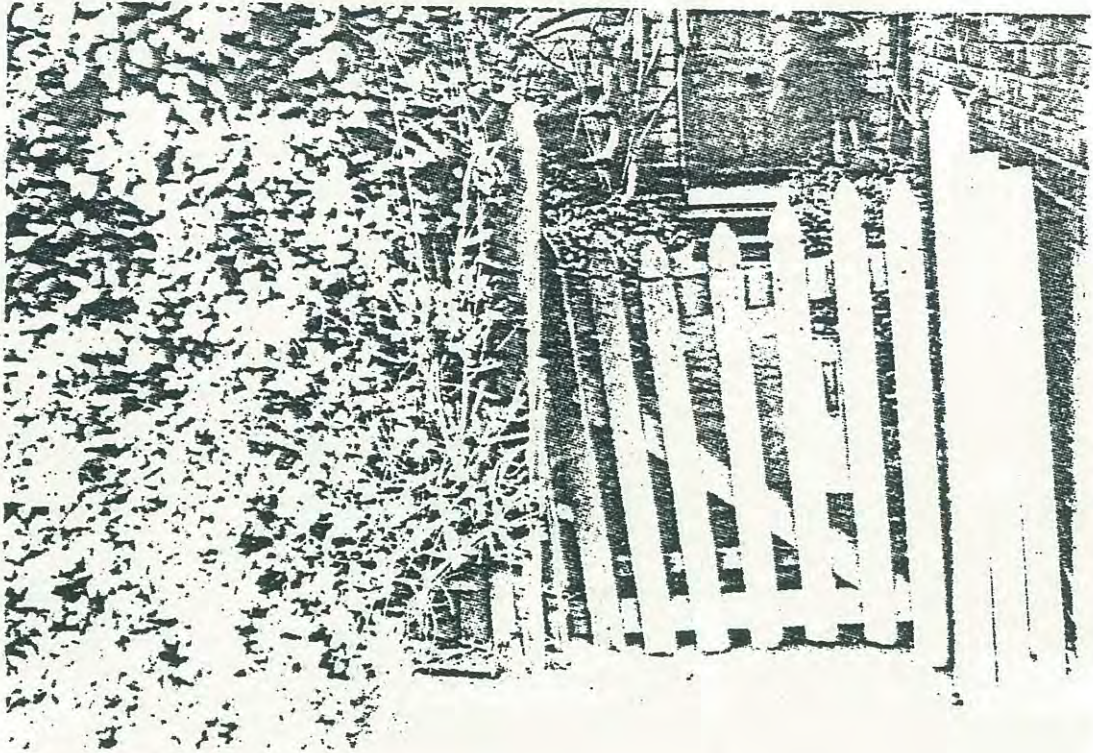
Fence, Gate at 46 Villiers St, 1883-4: 75x22 spade head picket, 73 space, 1200 high; posts 80x120, 1370 high.
