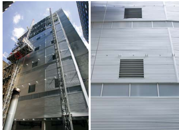
Figure 8: Vents for natural ventilation and windows for natural lighting of toilets located on the eastern façade, prior to installation of architectural cladding.
