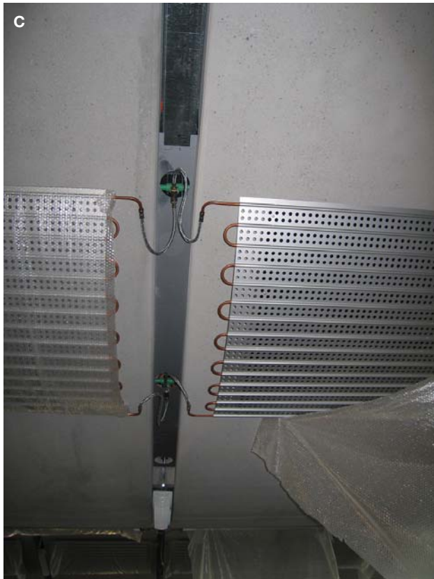
C: Perforated plate chilled ceiling panels showing copper piping connection, which continuously circulates water for radiant cooling via panels and the PCM storage tank in the basement.
