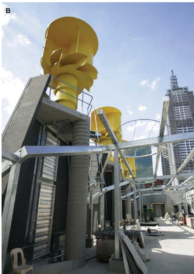
B: Mounted wind turbines showing the air extraction dampers (prior to connection to turbine).
