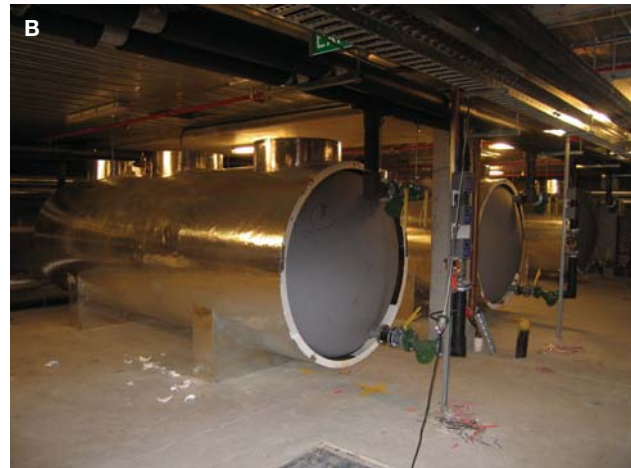
B. Bank of three PCM storage tanks located in basement (end insulation not fitted).
