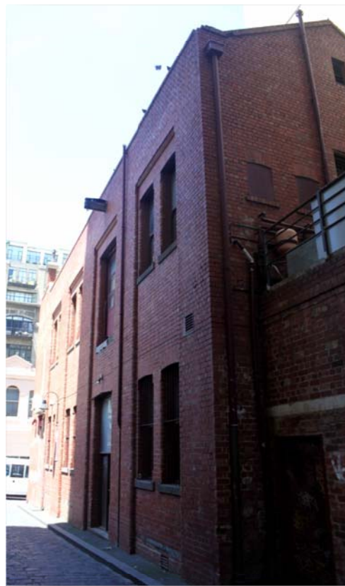
Figure 299 194-196 Little Lonsdale Street: rear and side elevation to lane, with early or original elements such as the cathead.
